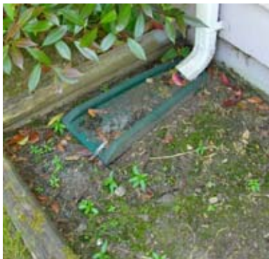
This splash block is discharging in a planter. Water trapped next to the building may end up under the home.
