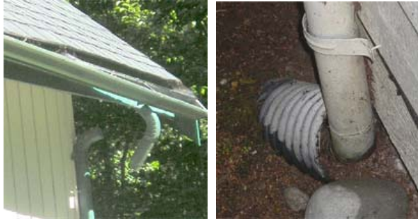
Gutter mounts failing and the downspout is disconnected. Keep downspout drains clear of mulch and debris.
