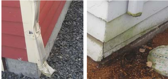
Repair any crushed or incomplete drains assuring they discharge away from the home.
