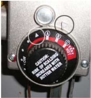
Gas water heater thermostats are easy to set, this one is too high. The 2 arrows should align.
